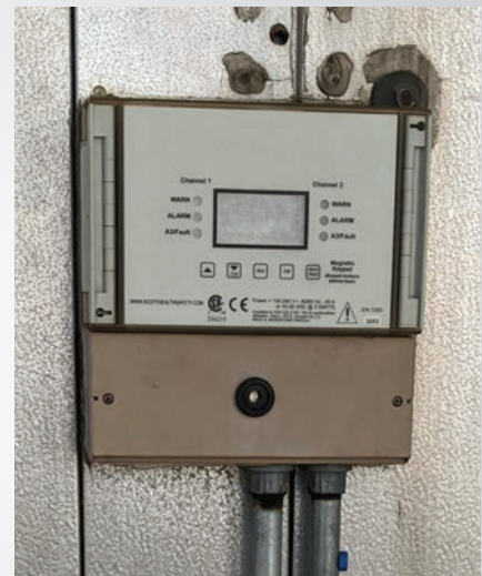
The ConsoliDator+ replaced this old degraded controller. The small display is hardly readable and it is exposed to the outside elements.
