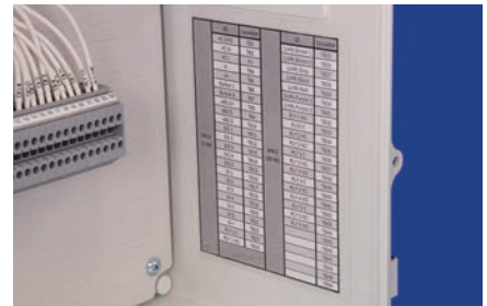
Wiring Table Attached Inside
