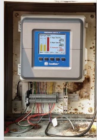
Enclosure opened showing wiring to ConsoliDator+
