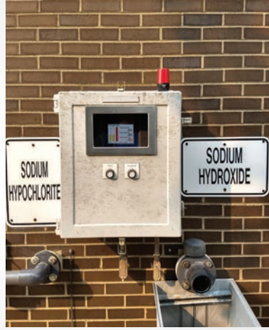
ConsoliDator+ installed in enclosure and mounted on wall outside the building
